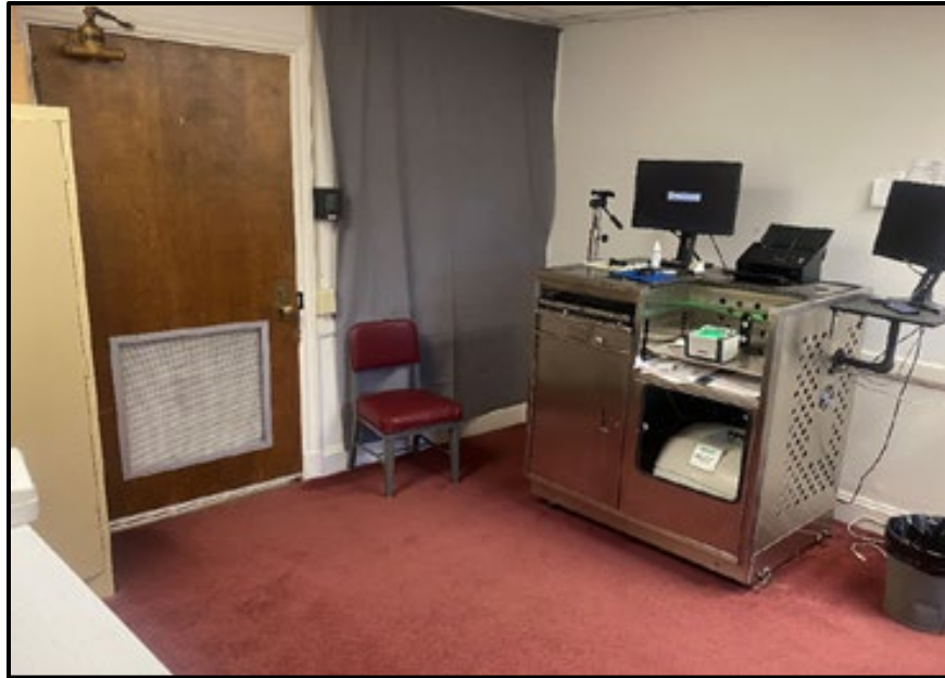
Location withheld – Prisoner processing room (carpeting drywall, unsecure door). Secure lock on door, but kickout vent leads to unsecure area.
