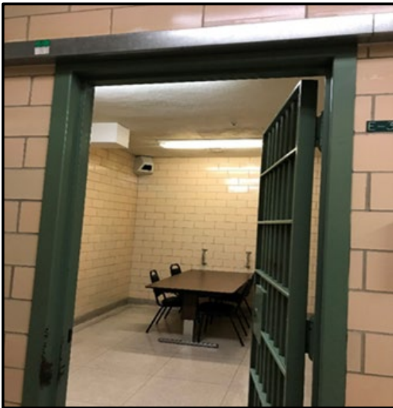
Washington, DC – District Court interview room: no prisoner/attorney separation, plaster ceilings, antiquated door does not provide sight/sound separation.
