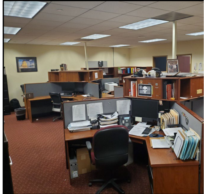
Camden, NJ – Worn carpet with trip hazards; outdated, deteriorating furniture needs to be replaced with more space-efficient systems furniture.
