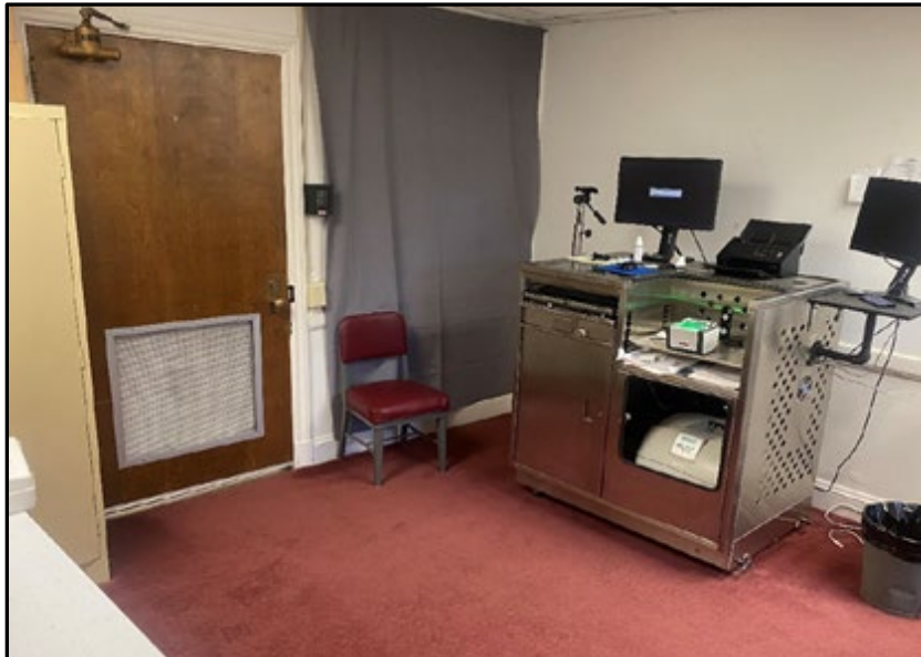
Location withheld – Prisoner processing room (carpeting, drywall walls, unsecure door). Secure lock on door, but kickout vent leads to unsecure area.
