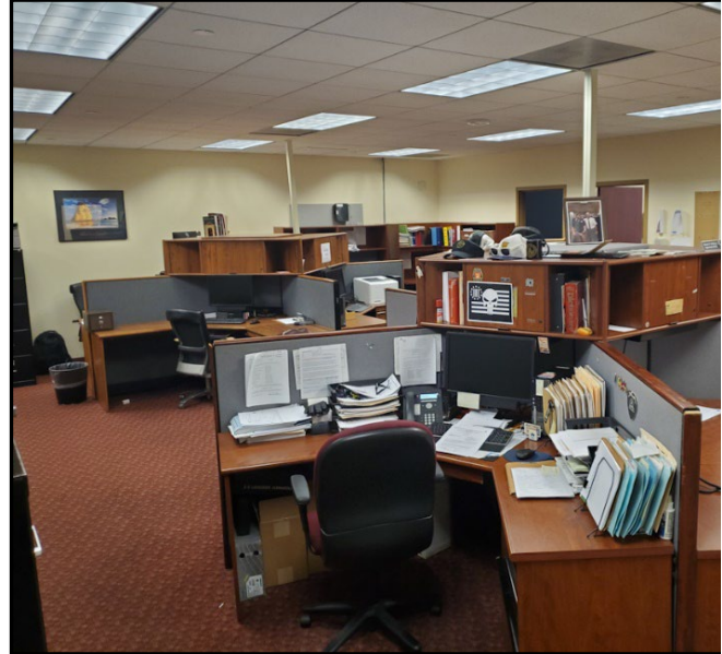
Camden, NJ – Worn carpet with trip hazards; outdated, deteriorating furniture should be replaced with more space-efficient systems furniture.
