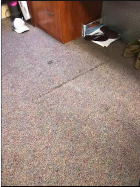
Washington, DC: Old carpet pulling up, trip hazard.
