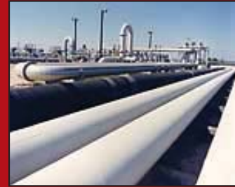
Crude Oil Pipeline at the SPR Bryan Mound Site, Freeport, Texas
