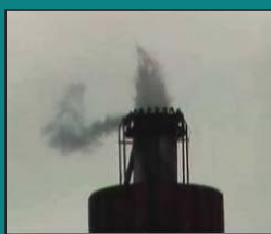
Poorly Operating Flare
